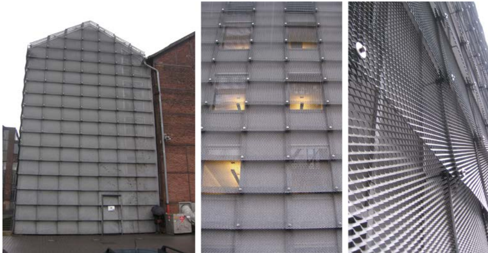
Fig. 2.6. Jahrhunderthalle in Bochum (Germany), façade refurbishment of industrial building transformed in concert-hall. Petzinka Pink Architekten, 2003
