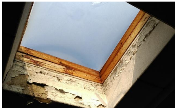
Figure 11: Picture of the damaged skylight.
