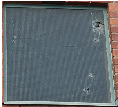
Figure 10: Picture of a broken window of the first floor.
