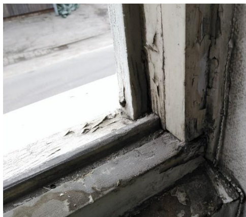
Figure 12: Picture of the windows with damage due to water infiltrations.
