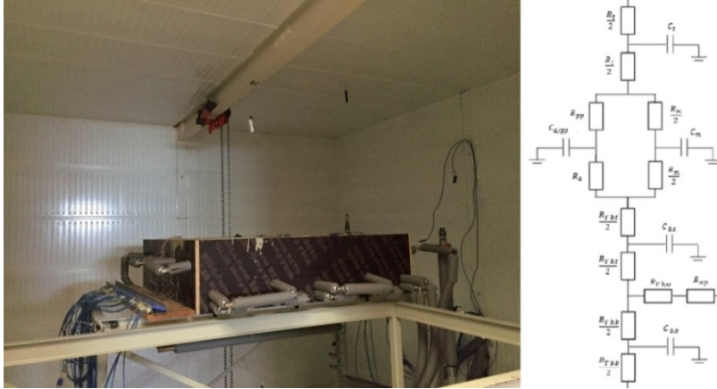
Figure 3.23. Experimental installation for TABS parametrization at KU Leuven and a proposed 6th order model for the characterization of an airbox filled TABS
