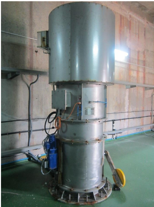
Figure 1. Turbo-generator module in NEREIDA MOWC wave power plant (Mutriku, Spain).
