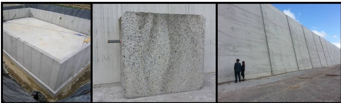
Figure 6.1: Kubik foundation and basement walls (left), a concrete block from the Punta Lucero dock (center) and the new Punta Sollana dock wall (right).
