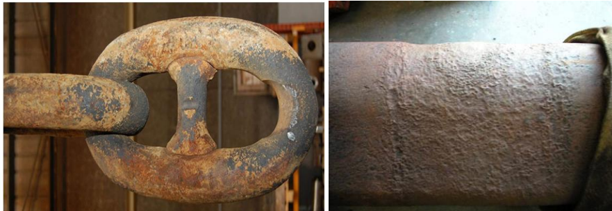
Fig. 2.6 Chain links showing severe wear in the inter-link contact (left) [51], and wear and pitting corrosion (right) [2]
