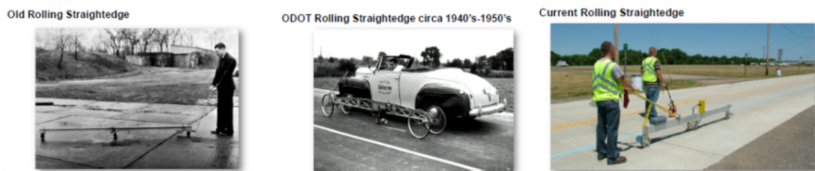
Fig. 3.62. Rolling straightedges. A) An old rolling straightedge, b) an ODOT rolling straightedge circa 1940s – 1950s, and c) at present.
