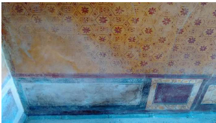
Fig. 10.11. Right wall of room I showing a widespread presence of efflorescences, where OR-1, OR-2, OR-3 and OR-4 measurements with high signal of S were performed.
