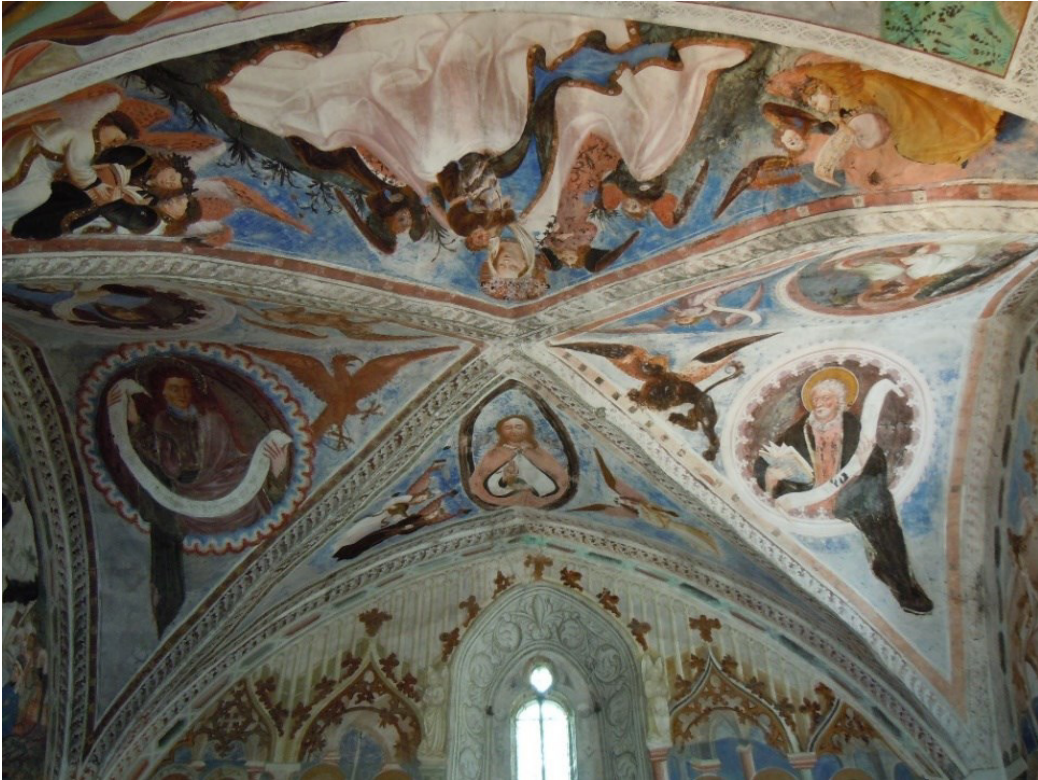
Figure 3.11: Vault of chapel where the blackening of paintings is evident.
