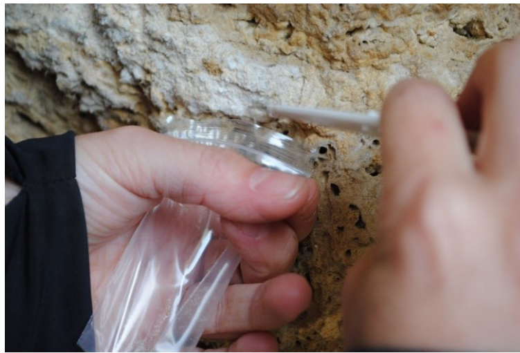
Figure 3.8: Sampling of salt efflorescences present in the structural walls.
