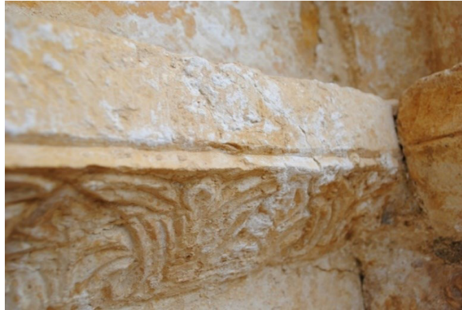
Figure 7.3: Evidence of salt crusts on the portal stone.
