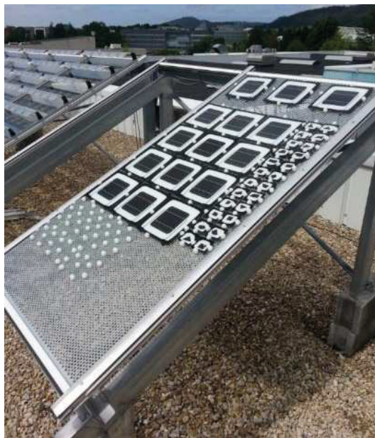
Figure 5-10. PV mono-modules exposed on the roof at TECNALIA's facilities.
