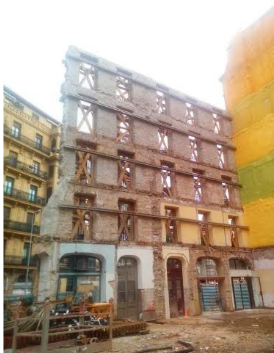
Figure 2. The elements of a typical load bearing stone wall, visible in detail during the building renovations of Easo street 1 and 2 cases.
