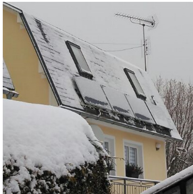
Figure 8. The single-family house for a typical winter season day, with the PVT collectors starting to melt earlier the snow compared to the PV module.
