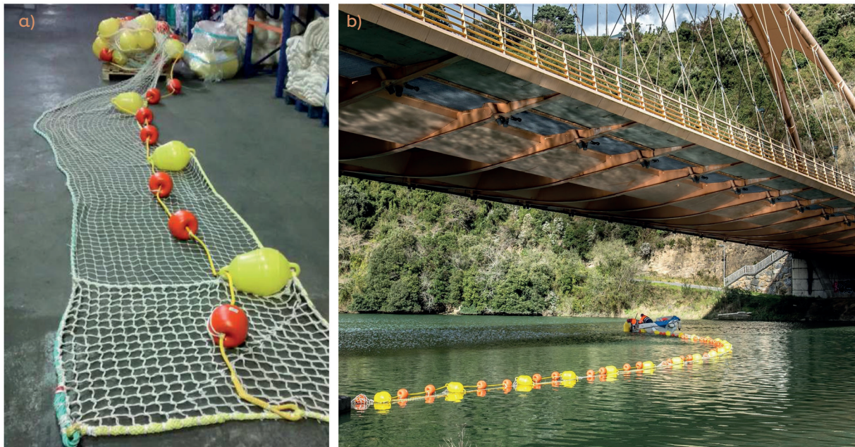
Supplementary Fig 5.17. Floating barrier for riverine litter collection. Floating barrier (a) and installation in Deba river (Gipuzkoa) (b).
