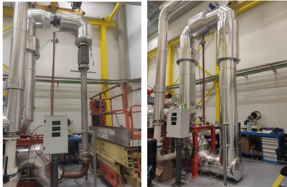
Figure 2. Thermal energy storage testing loop.
