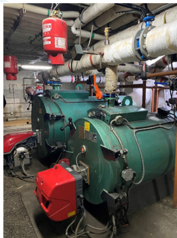
Figure 6. Boiler room located in the basement of Jauregizahar, 12 (Miriam Martínez, 2021).
