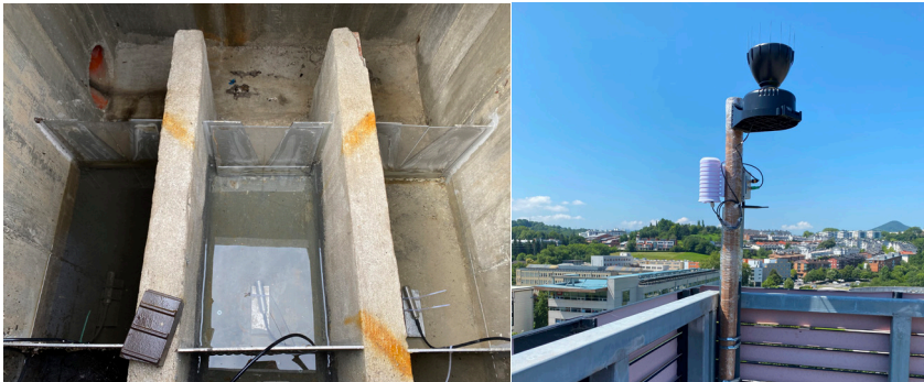
Figure 3. Three of the manholes built in Txomin-Enea. Weirs can be noted as well as the pressure sensors located in each manhole. Pluviometer installed on the roof of the School of Engineering of Gipuzkoa.
