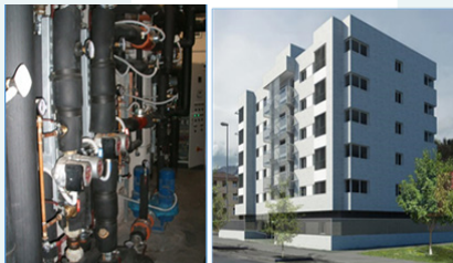
Figure 1. A partial view of the thermal facility and the building.
