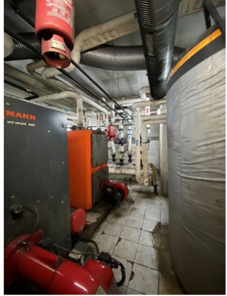
Figure 2. Boiler room located in the basement of Zumalakarregi 93 (Miriam Martínez, 2021).
