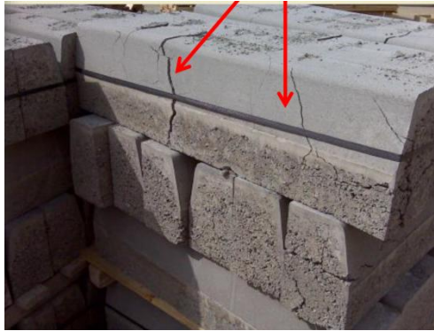
Figure 1: Effects of slag expansion in some kerbs.
