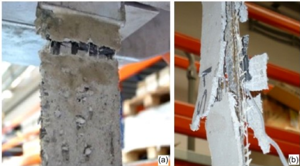
Fig. 5 Damage pattern in tensile tests: development of cracks in the vicinity of the aluminium plates in CTRM (a) and detachment of the mortar in SRG (b)
