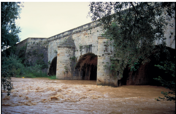
Fig. 30.11 The canal bridge of the Canal Imperial crossing the Jalón River. Photo: Rafael Araujo
