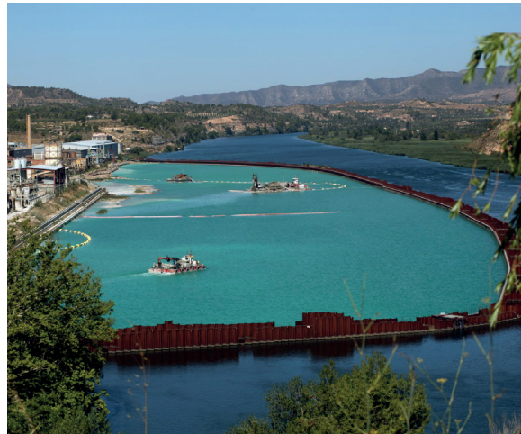
Decontamination work of sludge contaminated by the Ercros industry in Flix. Photo: Josep L. Sellart, with permission
