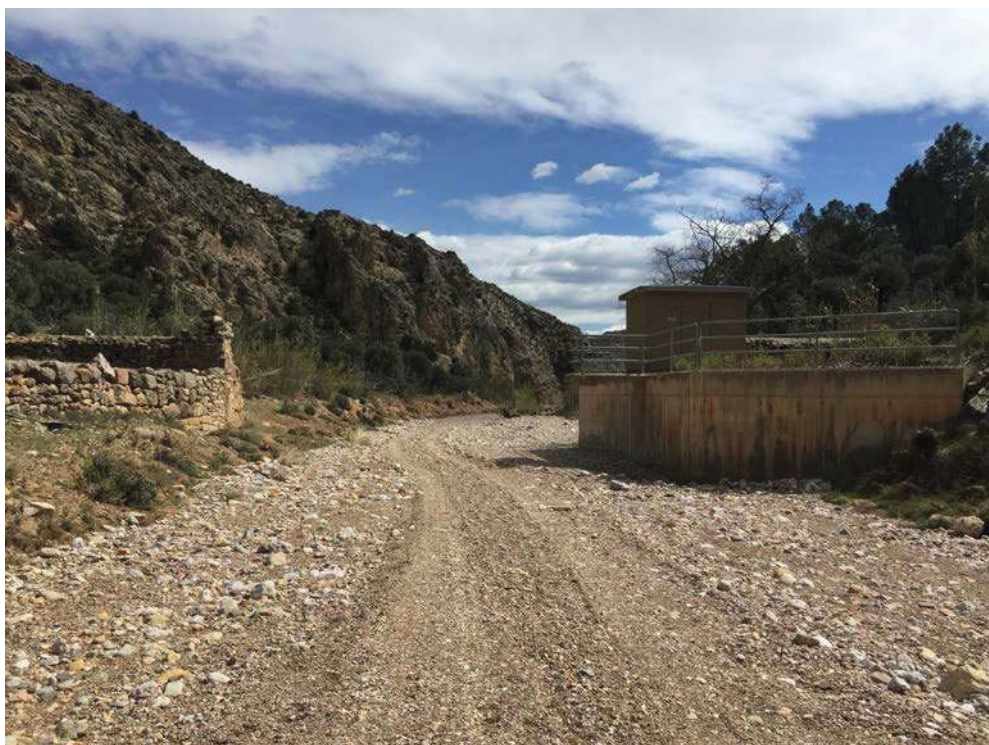
Figure 126. One of the very few gauging stations in the ephemeral network of the Ebro basin, that of the Seco River in Oliete (Teruel), built after the flash flood of 2013, which caused a fatality.
