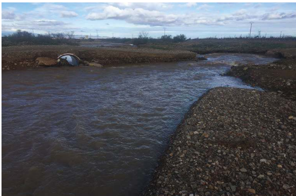
Figure 110. The flood in the Rambla de Cariñena, as a result of the storm Gloria episode (January 2020), destroyed the ford of the Virgen de Lagunas, rendering the only existing pipe under it useless. Apparently, this ford is illegal and it is the local owners who rebuild it after each flood.
