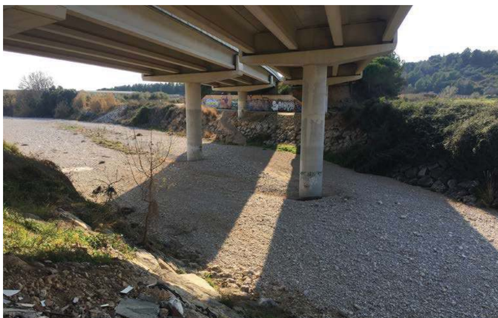
Figure 105. Bridge of the C32 over the Río Foix (Cubelles, Barcelona). The location of the pillars in the active channel could have been avoided.
