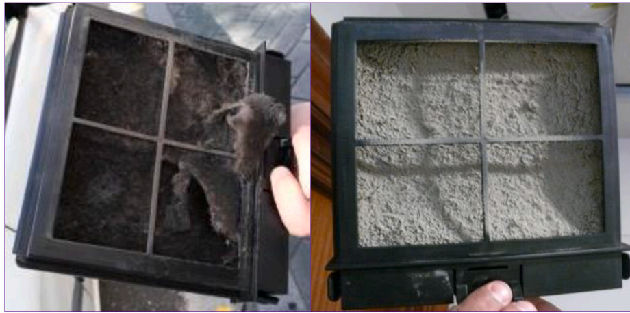
Fig. 8. Photos of the supply and extraction filters after the operating period.
