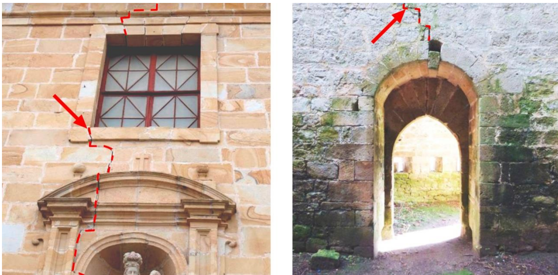
Figure 1. Cracks through the mortar in the Church of Markina and the Tower-House of Espinosa de los Monteros, in Spain.
