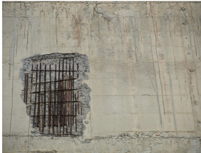
Figure 5. Vertical wall of the brutalist Carmelo Balda Fronton building in San Sebastián with some carbonatation damage. Photo: authors, 2019.
