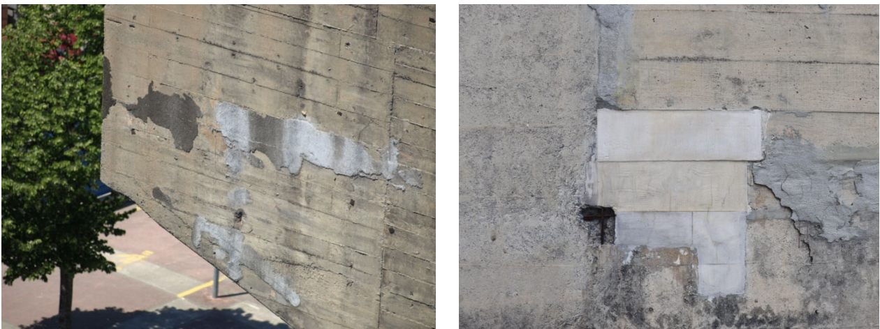
Figure 6. Current state of an isolated repair and a test with repair mortars of different tones on the brutalist Carmelo Balda Fronton building in San Sebastián. Photos: authors, 2019.
