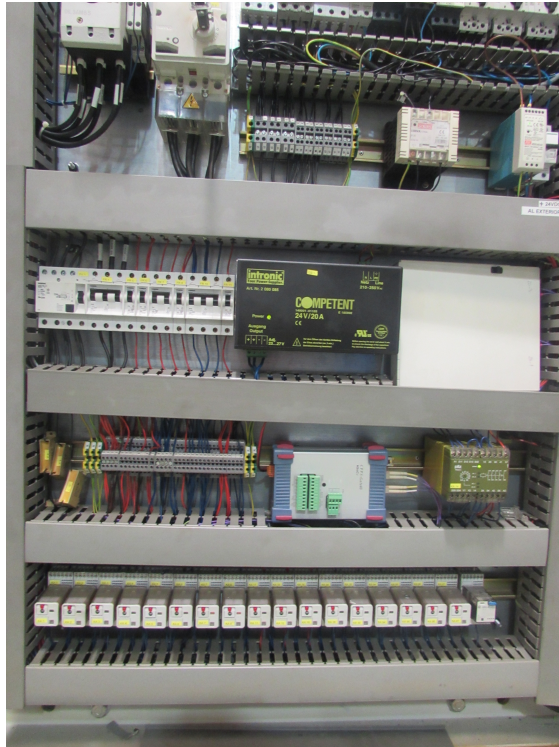
Figure 6.21: Picture of a CPPS Zynqbox installed in the industrial plant
