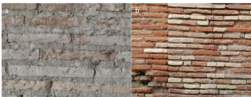
Figure 1. Appearance of the wall-building. a) With the mattifying veil; b) without an intense veil.
