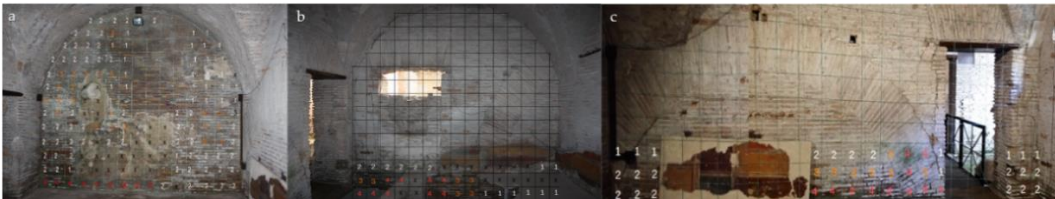
Figure 29. Modular grid installation in pre-Mithraeum room, with the Stage method values assignment. a) East wall; b) west wall; c) south wall.
