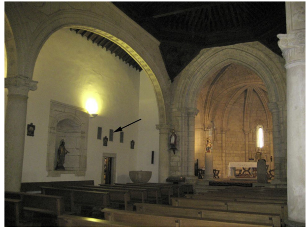
Fig. 2. NE corner of the church. The convection vents for the heating system are positioned at 3 m from the floor on the north wall of the north aisle.
