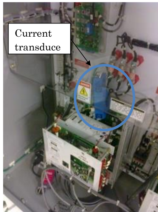
Figure 14. LEM HTA 100 S sensor installed in the test rig's electrical cabinet.
