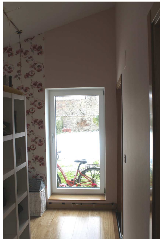
Figure 3.119: Window frame in dressing room, indoor IR image 13/03/2013.
