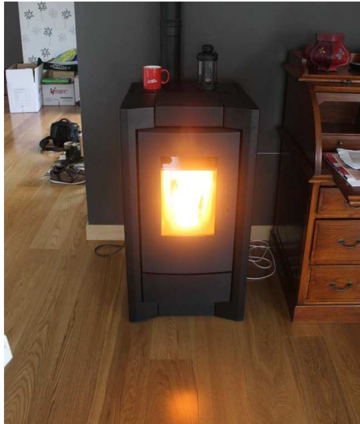
Figure I. 15. Detail the pellet stove heating on-use (right side).
