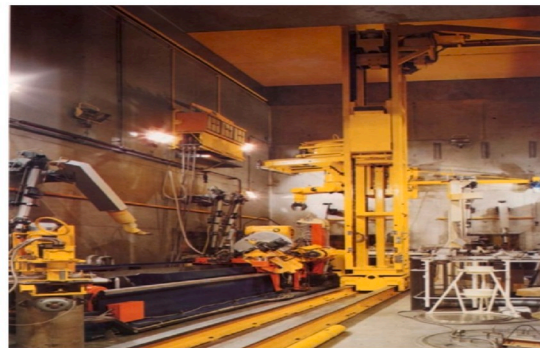
Example of decontamination room: waste treatment hot cell
