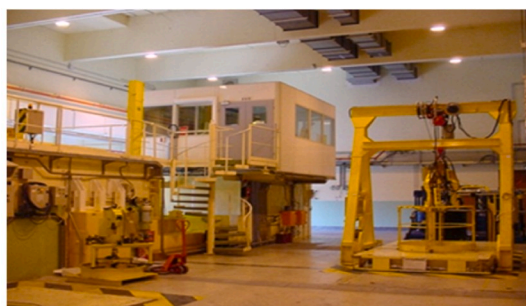
Example of equipment room : waste compaction process for ILW-LL waste
