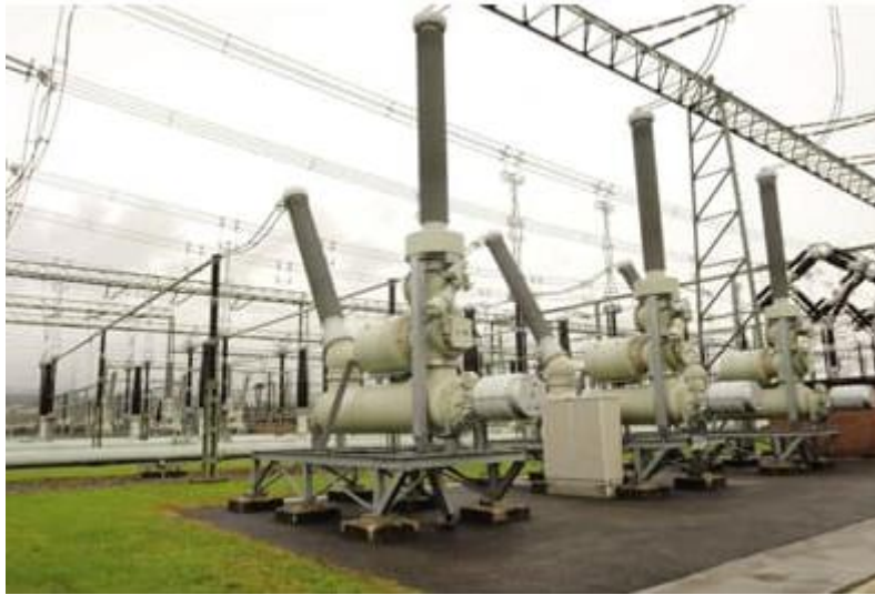
Figura 4: Subestación HIS ABB [7]
