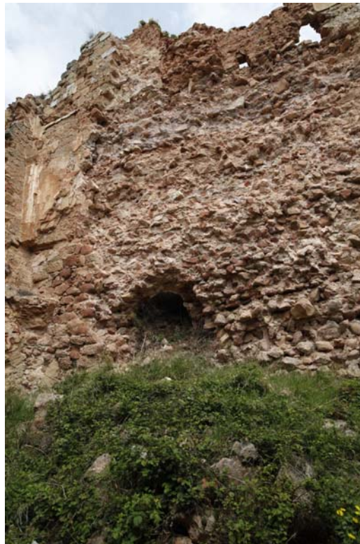
Image_28: Part of the northern wall will irregular surface
